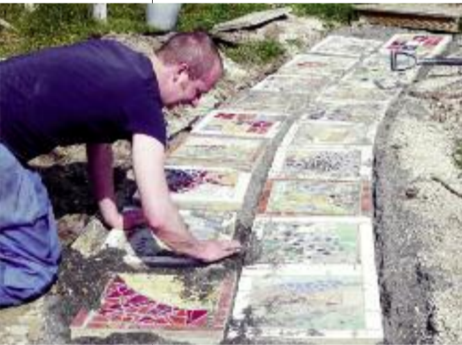
Laying a new path at Mountshannon made of mosaic panels created by community members.
